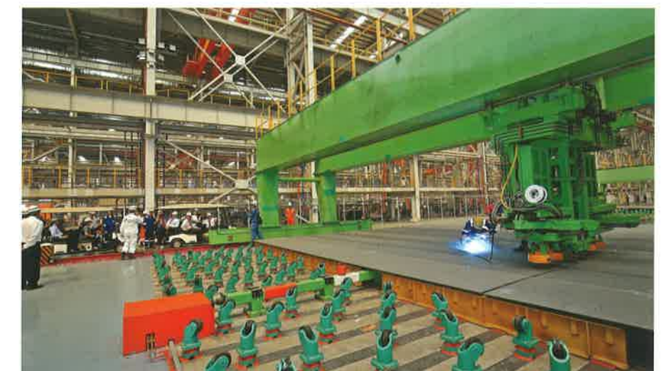
The 120,000-sqm facility included a fully-automated panel production line that delivers high quality welding precision and efficiency.
