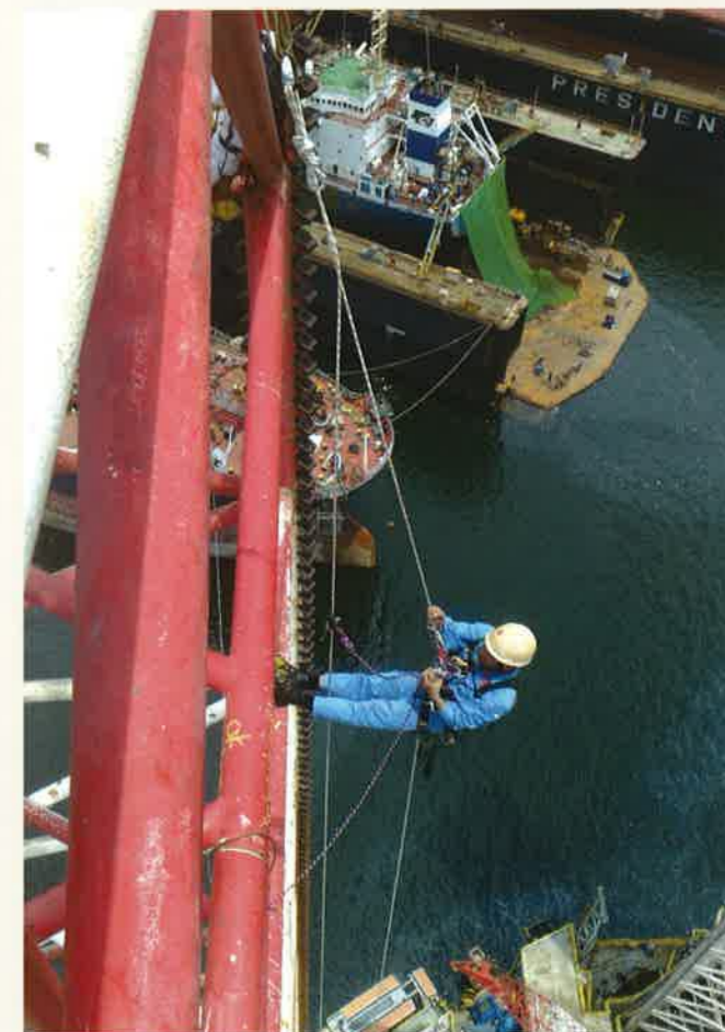
Rope Access Specialists accessing the water ballast tank and drilling rig jack-up structure for ultrasonic thickness measurement and close-up inspection.
