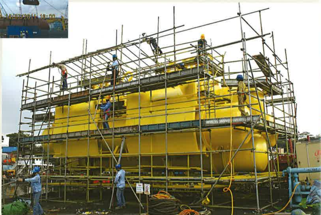
Refurbishment of Mid Water Arch which includes dry nitrogen refilling, part of the Abu FSO project.
