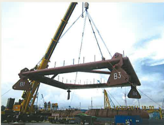
A 110-ton spreader beam being lifted by a 750-ton heavy lift mobile crane onto the 300' barge, part of the Montara Development Project.
